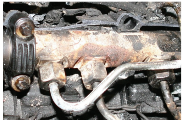
Fig. 13. Leakage Traces at a Connection Part
