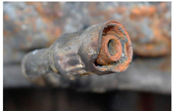
Fig. 7. Melted Pipe for Cooling of Turbo Charger
