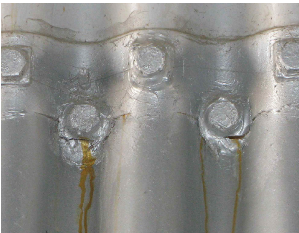
Fig. 2. Tearing and Water Leak at Bolted Connection
