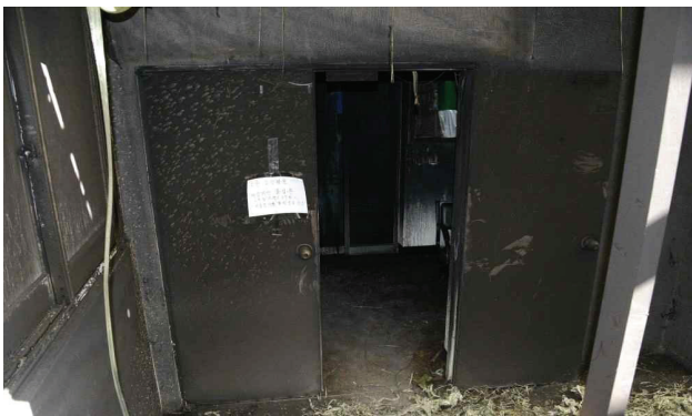
Fig. 13. Fire Door to Sejong Nurse Hospital in the Passageway on the 2nd Floor
