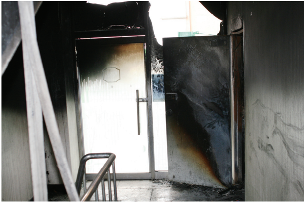
Fig. 7. Emergency Exit in the 3th Floor
