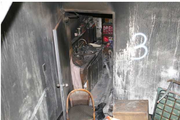
Fig. 8. Emergency Exit in the 3th Floor
