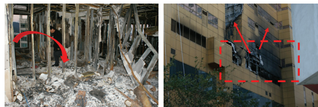
(a) Top Floor Fire Damage (b) Igniter Opening Status
