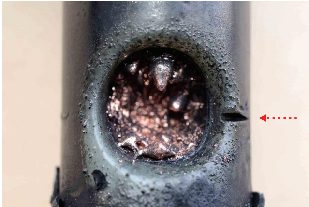
Fig. 10. Melted and Damaged Shape of Power Cable B-1
