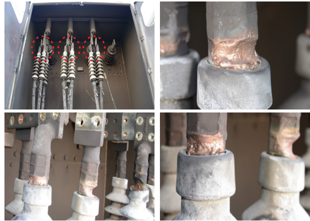
Fig. 5. Electric Arc of Cable Head
