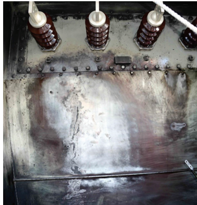
Fig. 6. Fire Pattern of Panel
