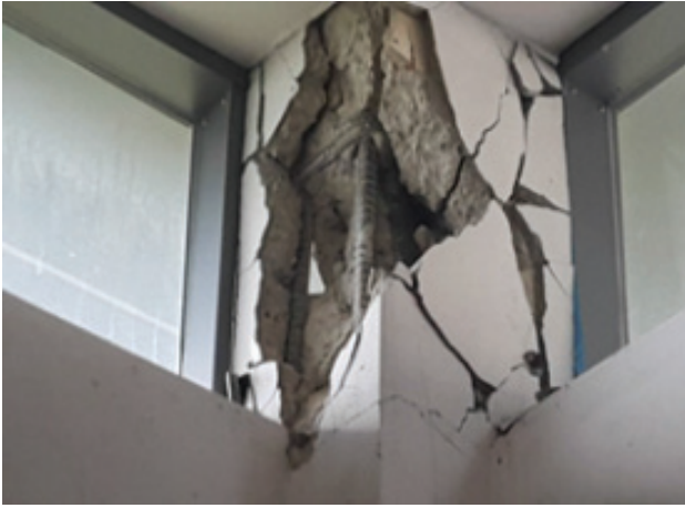
Fig. 1. Damage Examples Caused by the Gyeongju Earthquakes, 2016
